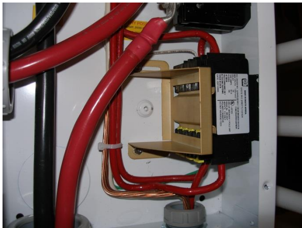
Din Rail mounted breakers
