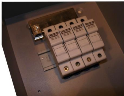
4 Touch safe fuseholders installed in an MNPV6
